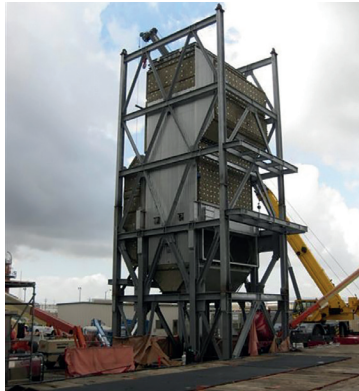
Figure 1: Heat exchanger for combustion air preheating.
